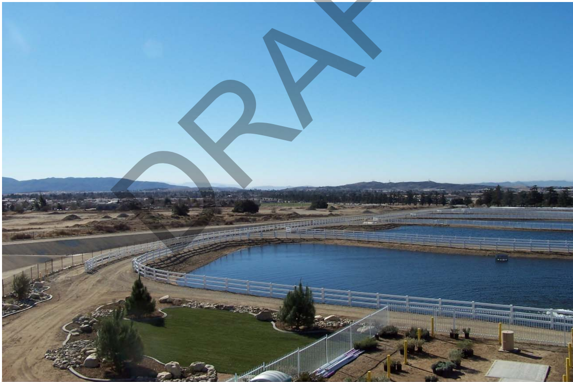
This is the Recharge Facility located on the south/east corner of Cherry Valley Blvd. and Beaumont Ave.
