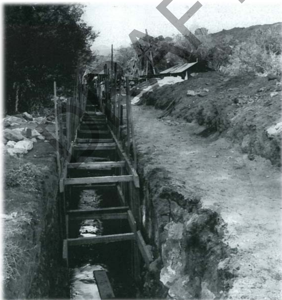
When well No. 2 was sunk north of Beaumont, it produced an adequate supply of water to the town, and a canal flume was built to bring it to Beaumont. The complexity of such an undertaking involved shoring up the canal wall, as can be seen in this photograph. (Courtesy of SGPHS.)
