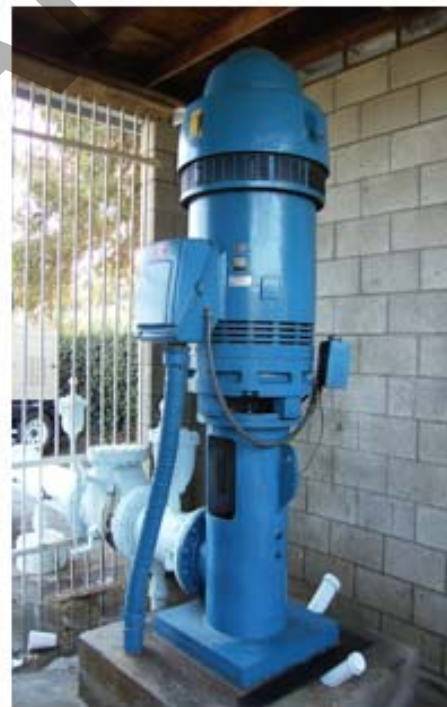
This is Well 1 today updated with a more efficient and modern pump.
