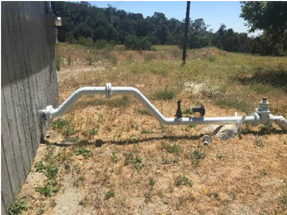
Well 20 Discharge Line
