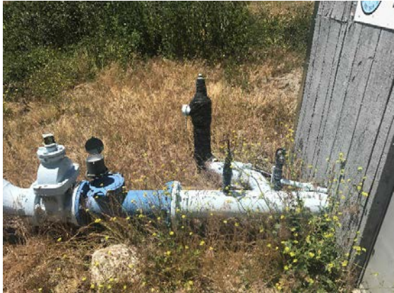
Well 19 Discharge Line
