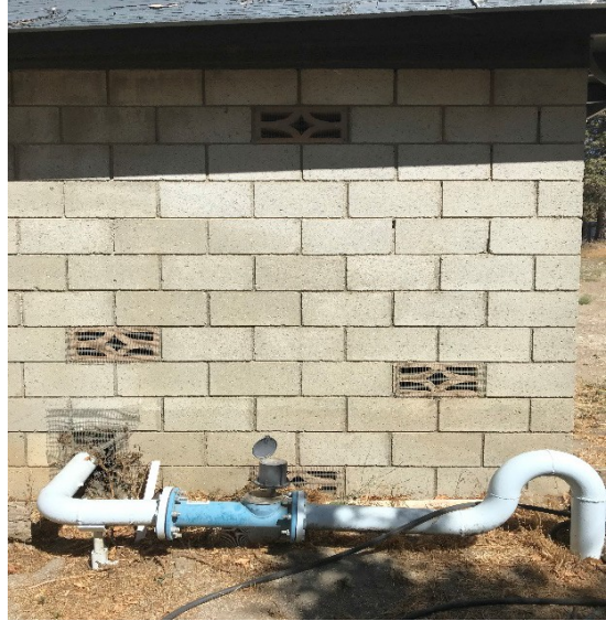
Well 11 Discharge Line
