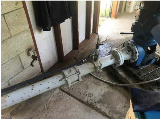
Well 12 Discharge Line
